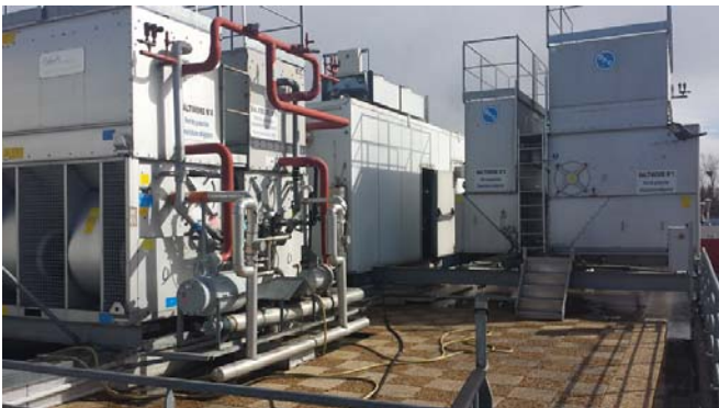
HP IMET unit and roof mounted condensers
