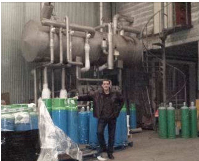
Benoît Duparc in front of the BP tank and recirculation pump
