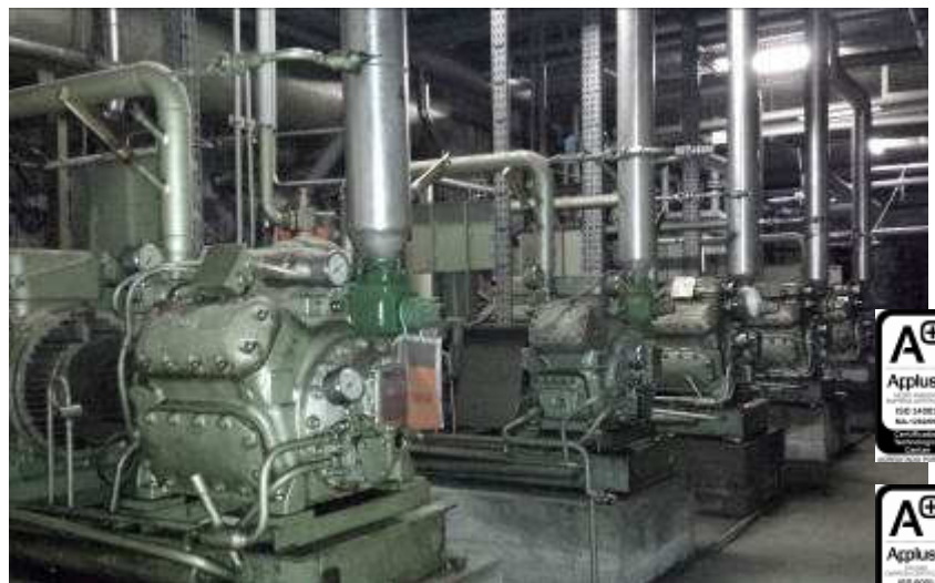
5 SAMIFI BABCOCK compressors 1986
